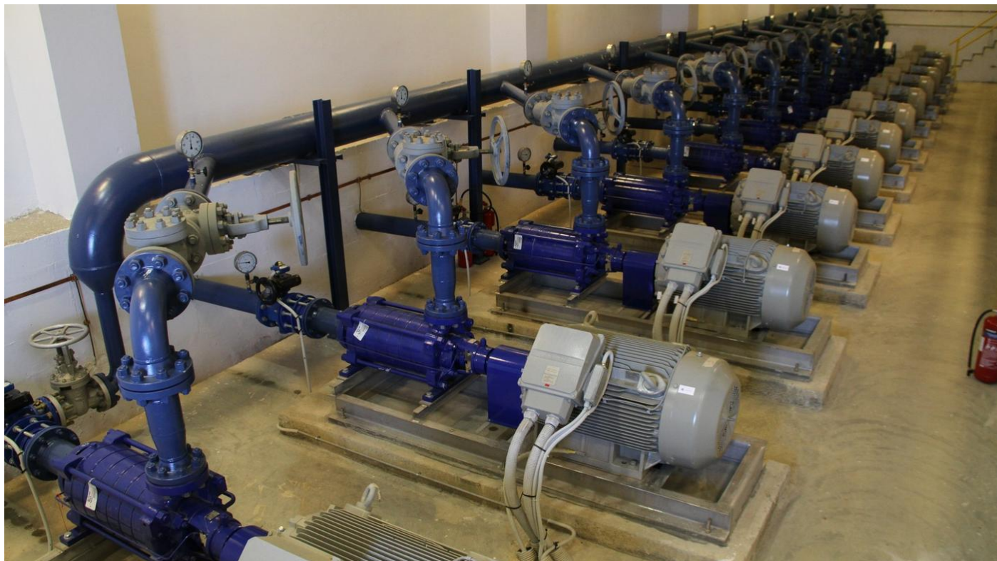
HPP Pumping Station, photo by www.4troxoi.gr
